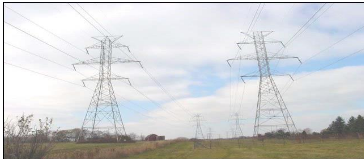
Figure 2: Two High Voltage Double-Circuit Transmission Structures
