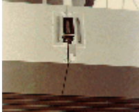
Photo of third floor walkway connections from below. See above photos for overall view of the third floor walkway. Note that from a distance, the fact that the third floor walkway was also distressed was not apparent. Also, the fireproofing cover box has been removed at this time.
