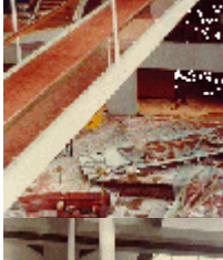
Photo of still-hanging third floor walkway. Note the free-standing stairs from the second to the third floor in the background. With its columnless design, the stairs seem to be floating in air. The lobby was indeed a masterpiece of architecture and engineering which, had it been executed properly, would have provided its owners with profit and the public with a stunning atmosphere for years.
