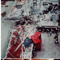
Photo of walkway sections taken from second floor opening. Walkway sections have been moved from their original positions during the attempt to extricate those trapped in the wreckage.
