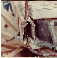
Photo of one of the walkway cross- beams, lying on the floor of the lobby. This is one of the fourth floor beams, as evidenced by having two bolt holes drilled through the beam. The second floor beams had a single rod hole.
