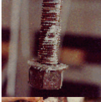
Close-up photo of the hanger rod threads, washer and supporting nut. Note the deformation caused in the washer as the beam slipped around it.
