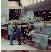
General view of the lobby floor, during the first day of the investigation.
