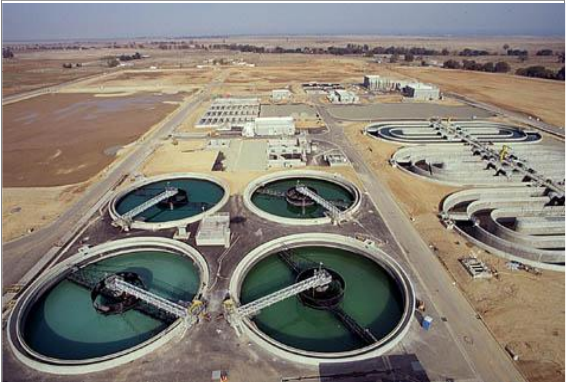
Water Treatment System
