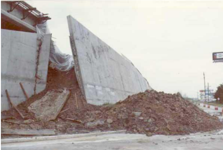
Failure by sliding
