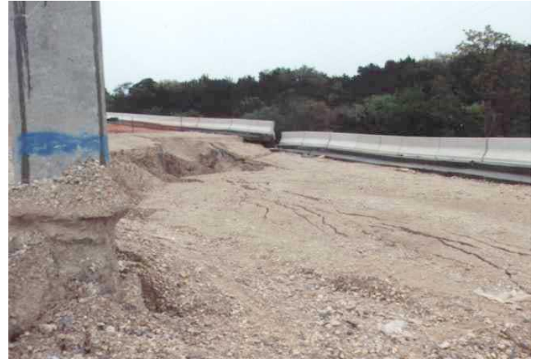
Failure by settlement
