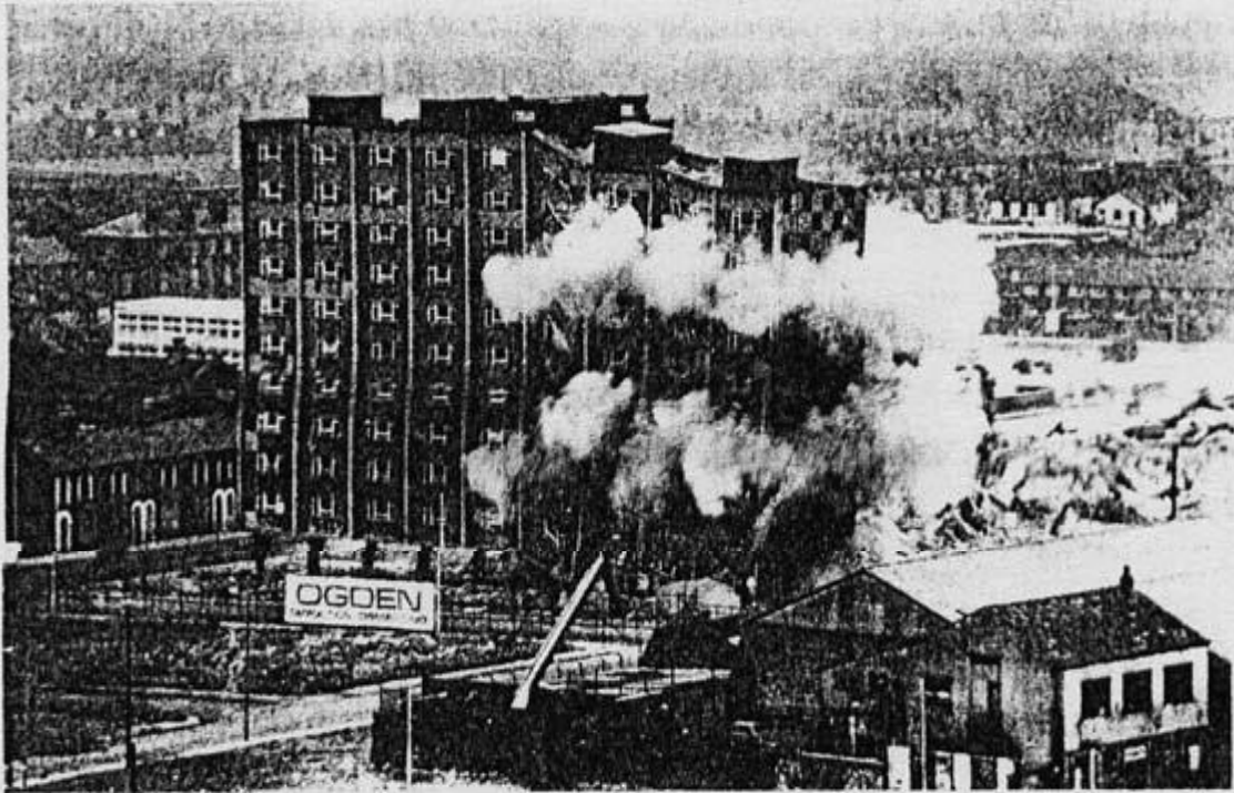
PLATE 1. Failed Utopia. The last wing of a massive complex of flats embodying many officially recommended design features such as 10 storeys poised on concrete stilts, internal corridors, flat facades and flat roofs. When built, a brochure was circulated to local authorities showing it as a Utopian ideal to be imitated. Yet it proved unsalvageable and hundreds of imitators were also condemned to a short life. (Eldon and Oak Gardens, Birkenhead)
