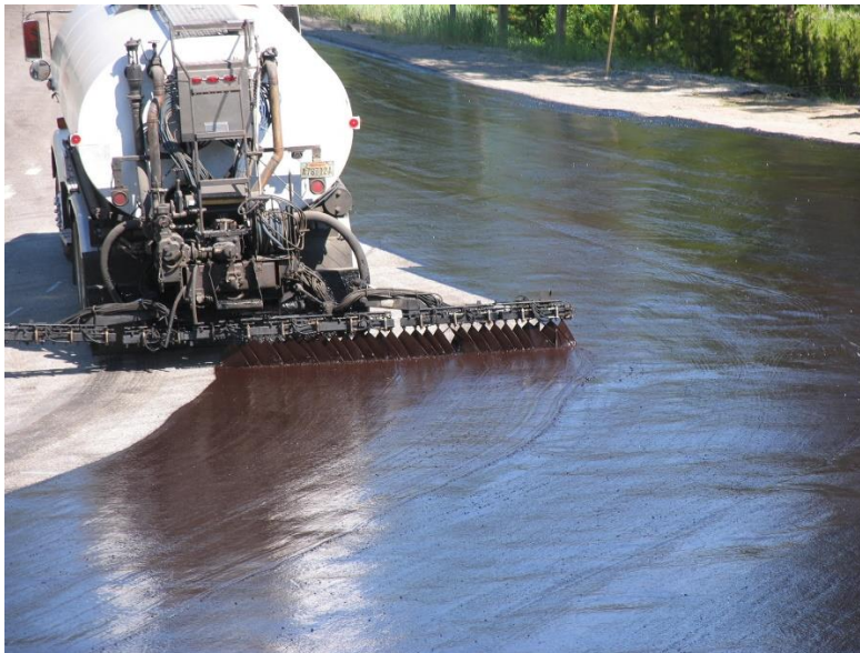
Figure 6: Freshly placed asphalt emulsion for a bituminous surface treatment; notice that the application rate is higher than that for a tack coat.
