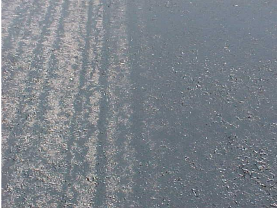
Figure 3: Poor tack coat (shown in the left half of the photo) vs. a good tack coat (shown in the right half of the photo). Notice the streaky coverage of the poor tack coat and the near complete coverage of the good tack coat.
