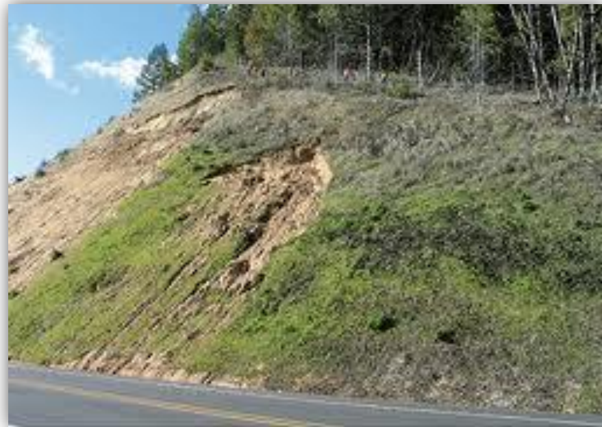
Signs of slope instability
